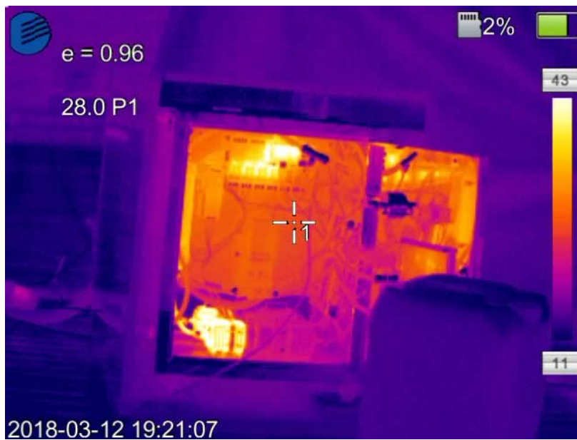
Fig.4 An infrared image of the Sewage treatment equipment (for whom concerns)
